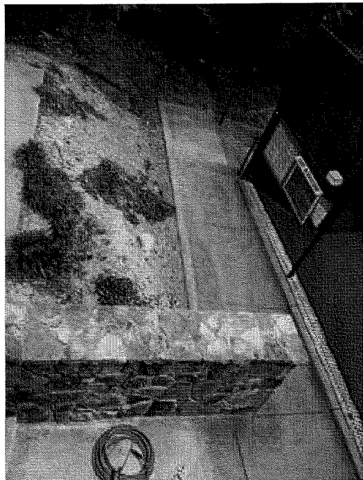
View from above the area adjacent to the tennis courts before renovation.
